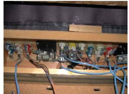
Figure 5. My goal was to avoid soldering. The spade plugs look great, but they honestly don't make a very good connection—another example of what not to do.
