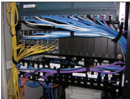
Figure 2. The Citylink fibre (yellow cables) is converted to copper (blue) for distribution to clients.
