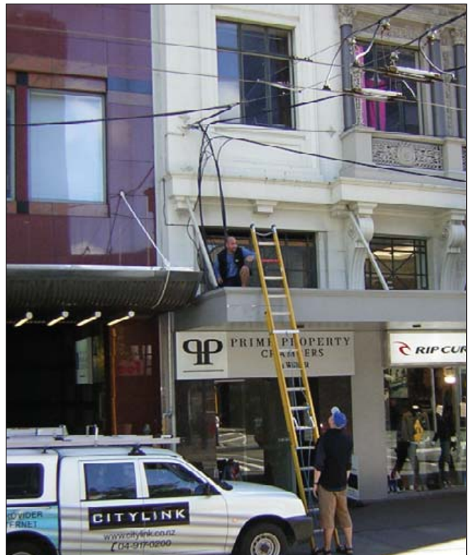
Figure 4. Cables coming off overhead trolley bus supports to a junction point on a building veranda. The ability to exchange huge files at no cost helps local businesses save money and offer new services.
