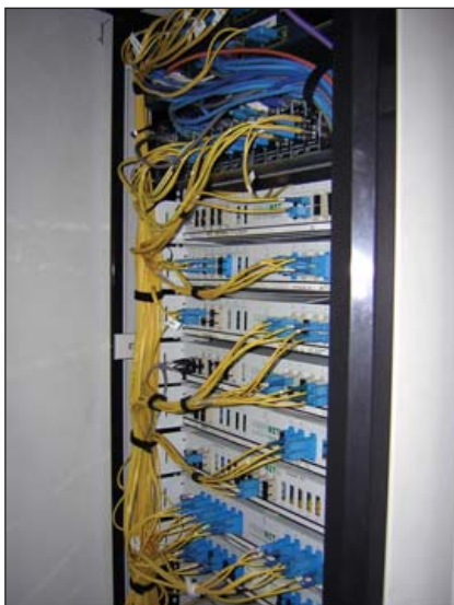
Figure 3. A typical fibre switching point, as found in many PABX rooms around Wellington.
